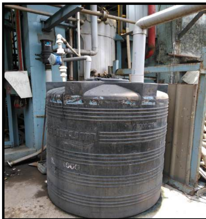
Photographs of Rain water harvesting system
