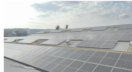
Rooftop Solar Panel
